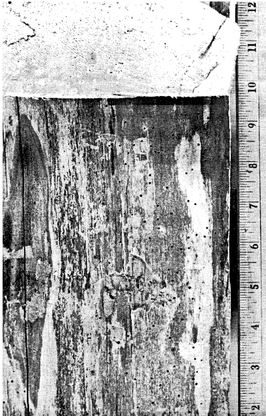
FIGURE 4-21 Anobiid Damage Showing Insect Exit Holes
