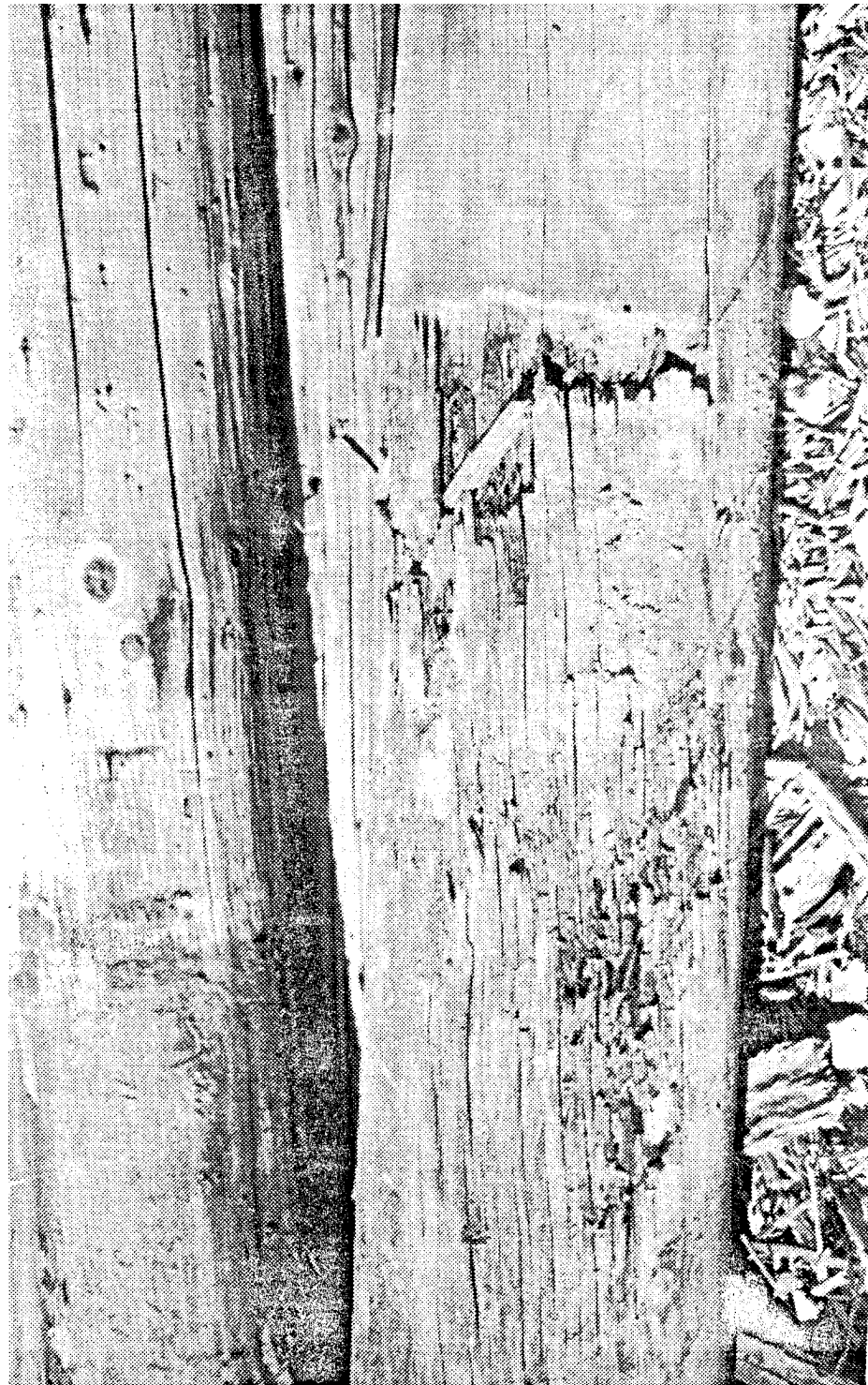
FIGURE 7-2 External or Surface Decay is Most Common at the Ground Line
